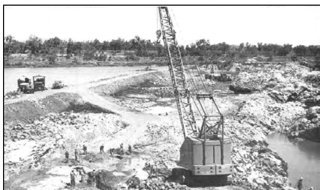
Rock excavation at Bandicoot Bar, protected by a temporary upstream levee. Photo courtesy Christiani & Nielsen
